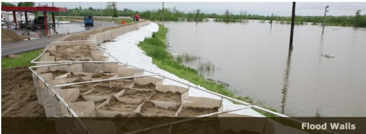
Fig. 2: Increasing the water flowing capacity of the stream by placing sand filled Geo-bags
